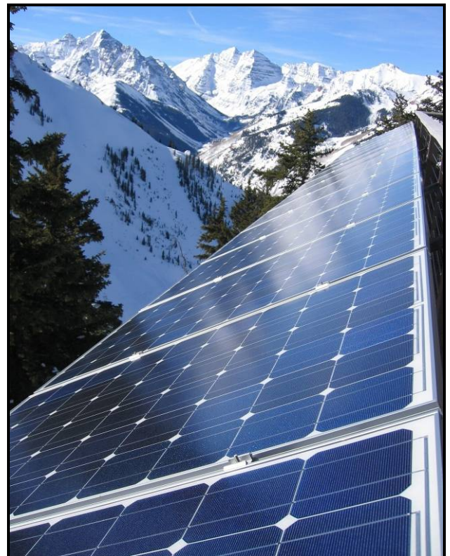
Aspen solar panels (Photo courtesy of ASC)
