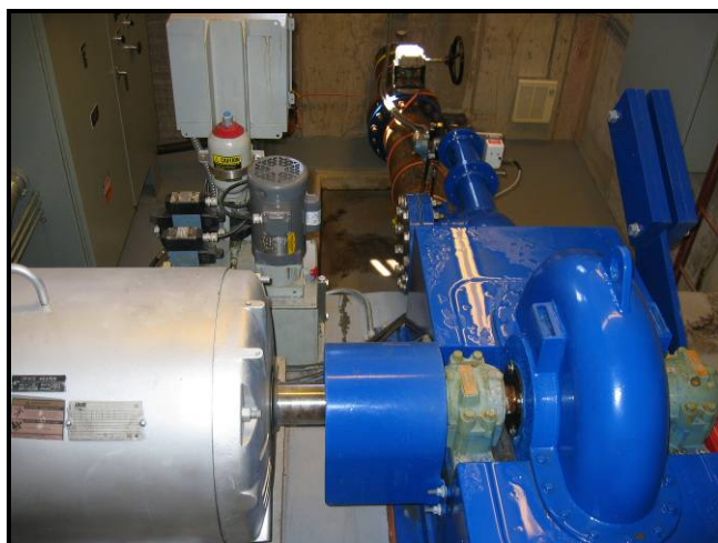
Turbine and generator (Photo courtesy of ASC)
