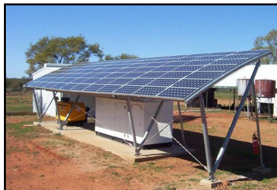
Solar PV roofs take advantage of Queensland Parks ample sunlight. (Photo courtesy of Queensland Environmental Protection Agency)
