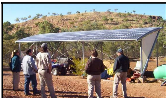
Solar panels both generate electricity and provide shade. (Photo courtesy of Queensland Environmental Protection Agency)
