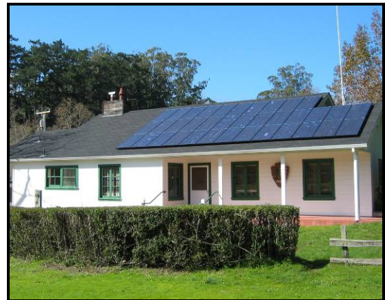
Solar panels cover much of this NPS office roof. (Photo courtesy of Steve Butterworth)
